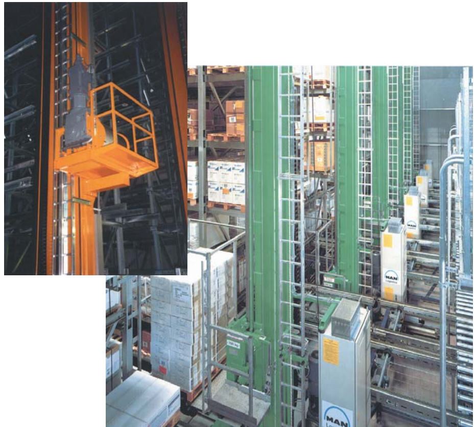
Rack access system with helical gear motor, encoder and brake with hand ventilator, motor fed from inverter
